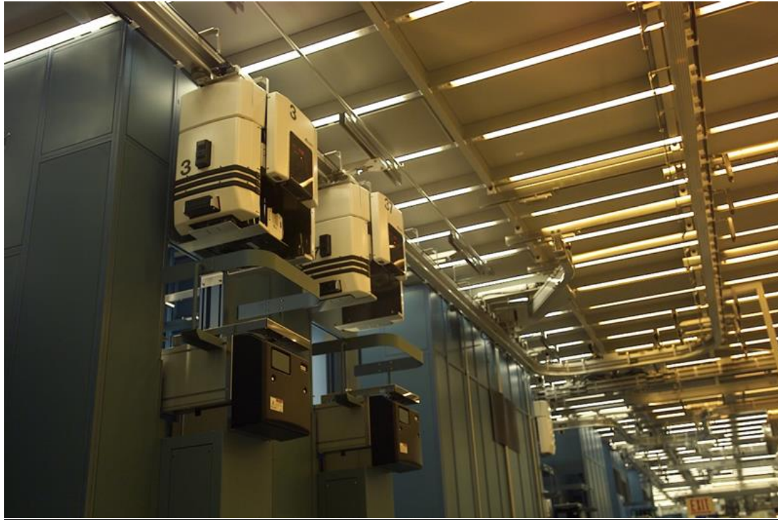
Figure 4. Robotic system moves wafers inside enclosed containers (FOUPs).
